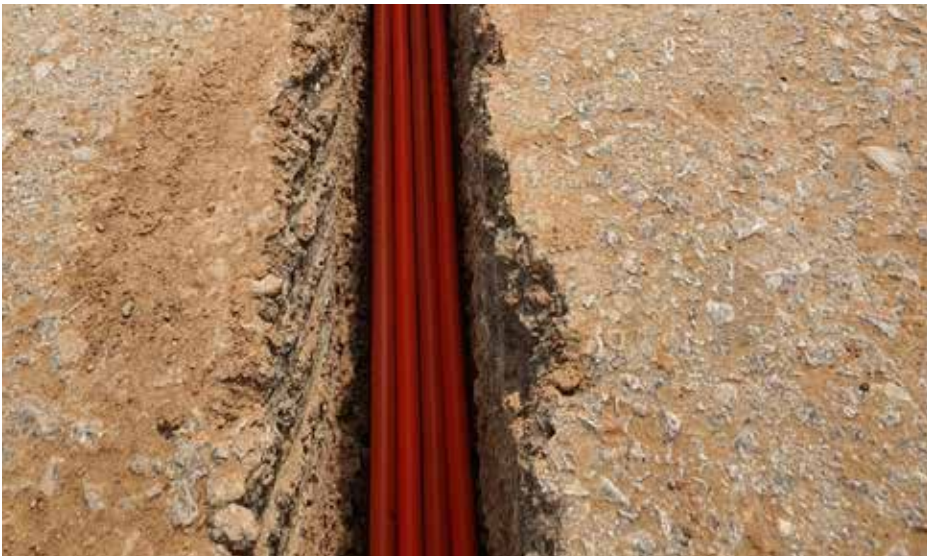
Project: Long Distance Fiber (LDN) Client : Ministry of Interior (MOI) Consultant: NEC Location : Azzulfi
